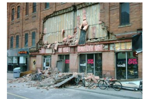
4 Lalani - collapse of the façade
